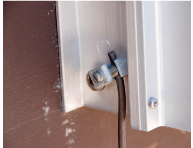
Close-up of an external grounding electrode terminal.
