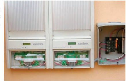
Two inverters and their AC combiner, with breakers.
