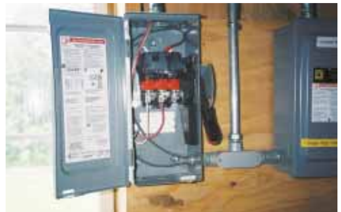
Not to code: grounded conductor switched.
