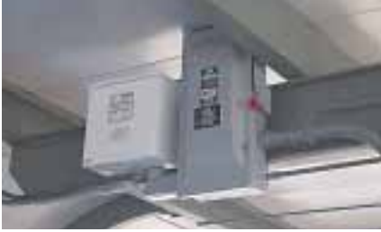
Not to code: disconnect 10 feet in the air.
