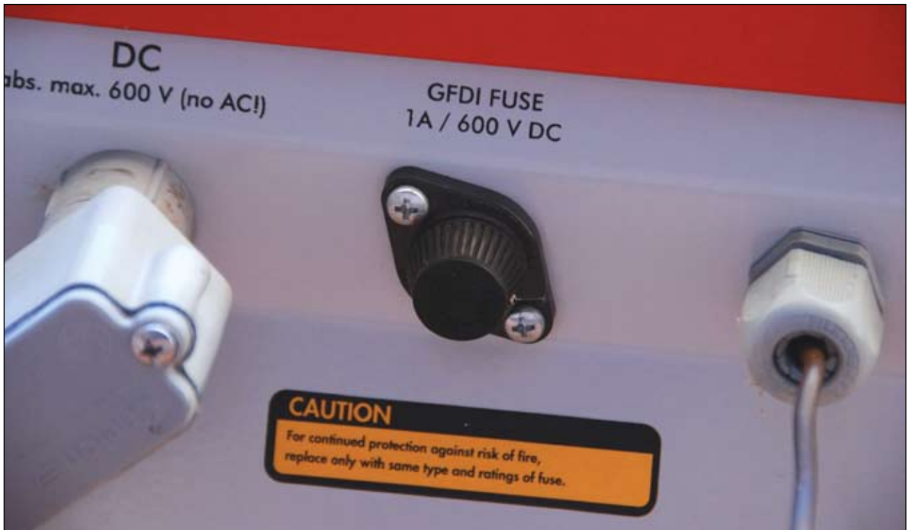
Photo 4. Ground-fault fuse on high-voltage inverter
