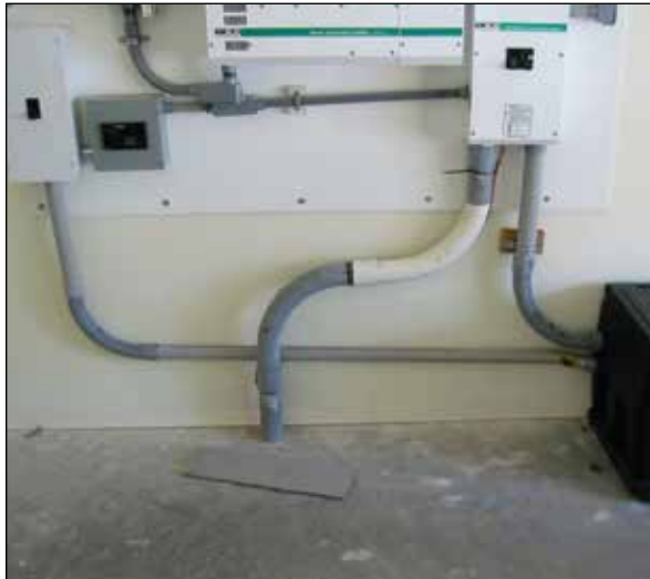
Photo 2. Battery disconnect adjacent to battery enclosure article to cover completely and that article will be in a forthcoming IAEI News (photo 3).
