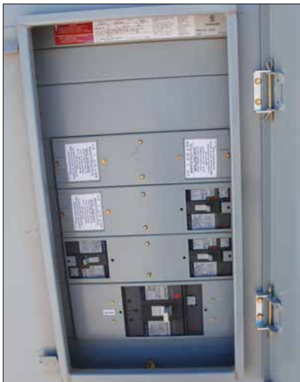
Photo 3. Clarifications coming for load-side connections.
