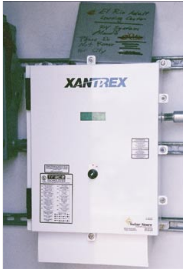
Photo 8. 15 kW 3-phase utility-interactive inverter
