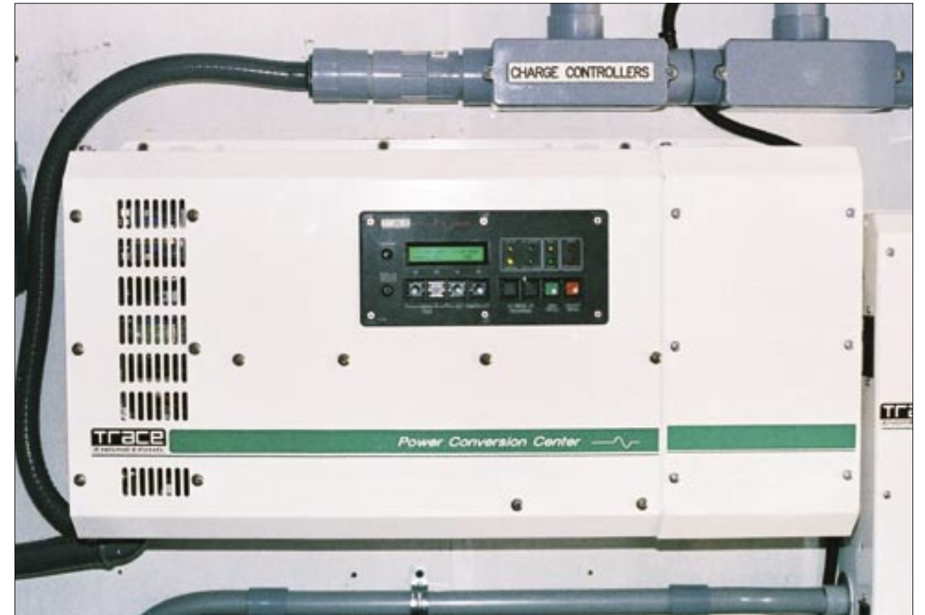
Photo 9. 4 kW stand-alone inverter
