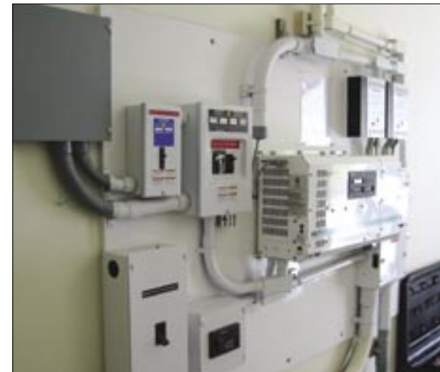
Photo 6. Off-grid PV power system
