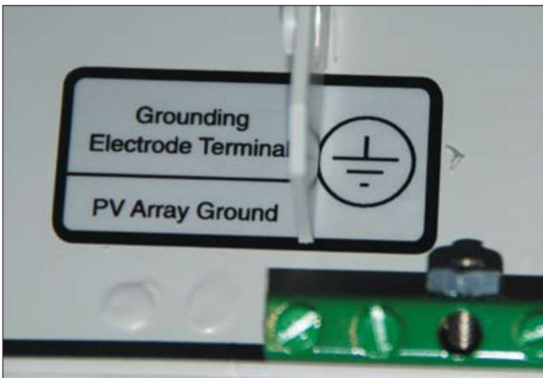
Photo 2. Grounding bus bar
