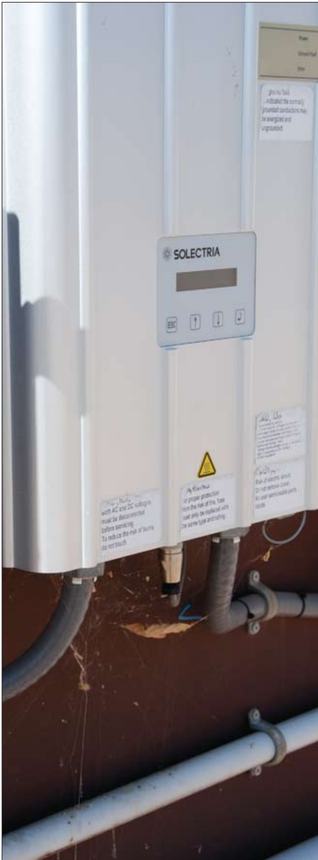
Photo 6. Grounding electrode conductors permanently attached in conduit
