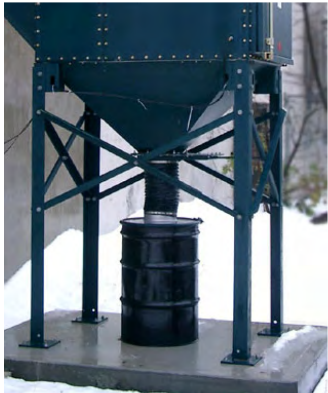
Storage drum prevents dust from backing up in the hopper and creating an explosion hazard.
