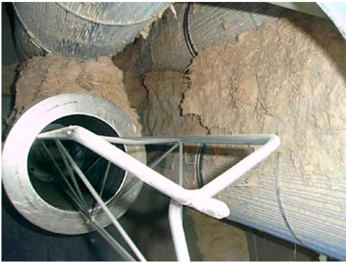
Figure 4: Example of horizontally-mounted dust collector filters
