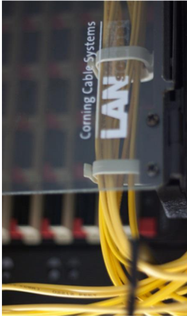
NMSU fiber optic cable
