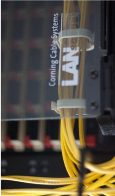
NMSU fiber optic cable
